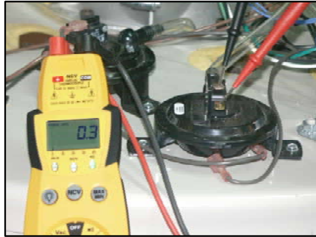
Continuity Test With Ohm Meter BTH 120 - 250 Blocked Exhaust Switch
