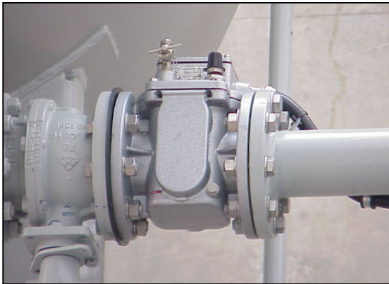
Figure 34 – Photograph of a Buchholz Relay.
