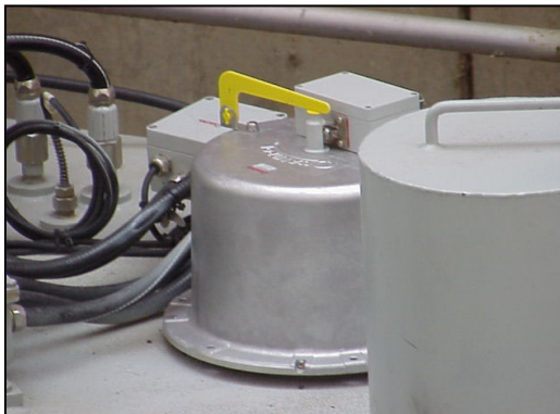
Figure 30 – Photograph of a Pressure Relief Device.
