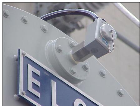
Figure 41 – Photograph of a Bladder Failure Relay.
