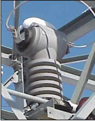
Current Transformer in Switchyard.
