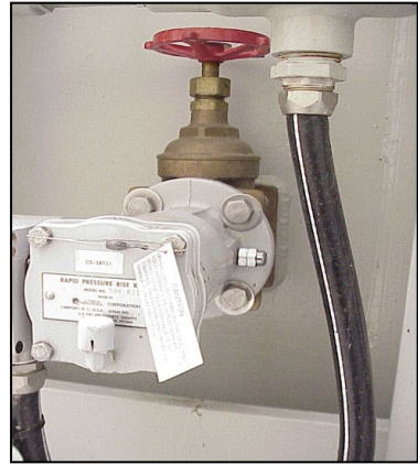
Figure 32 – Photograph of a Sudden Pressure Relay.
