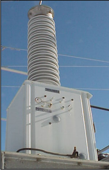
Potential Transformer in switchyard.
