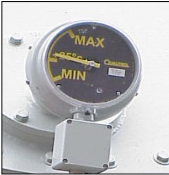
Figure 28 – Conservator Oil Level.
