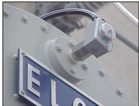
Figure 41 – Photograph of a Bladder Failure Relay.
