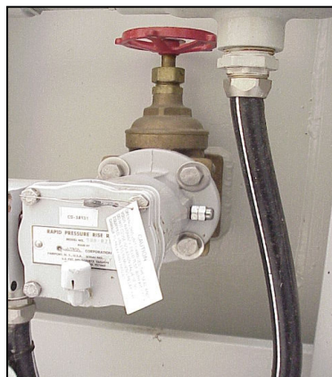
Figure 32 – Photograph of a Sudden Pressure Relay.
