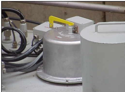
Figure 30 – Photograph of a Pressure Relief Device.
