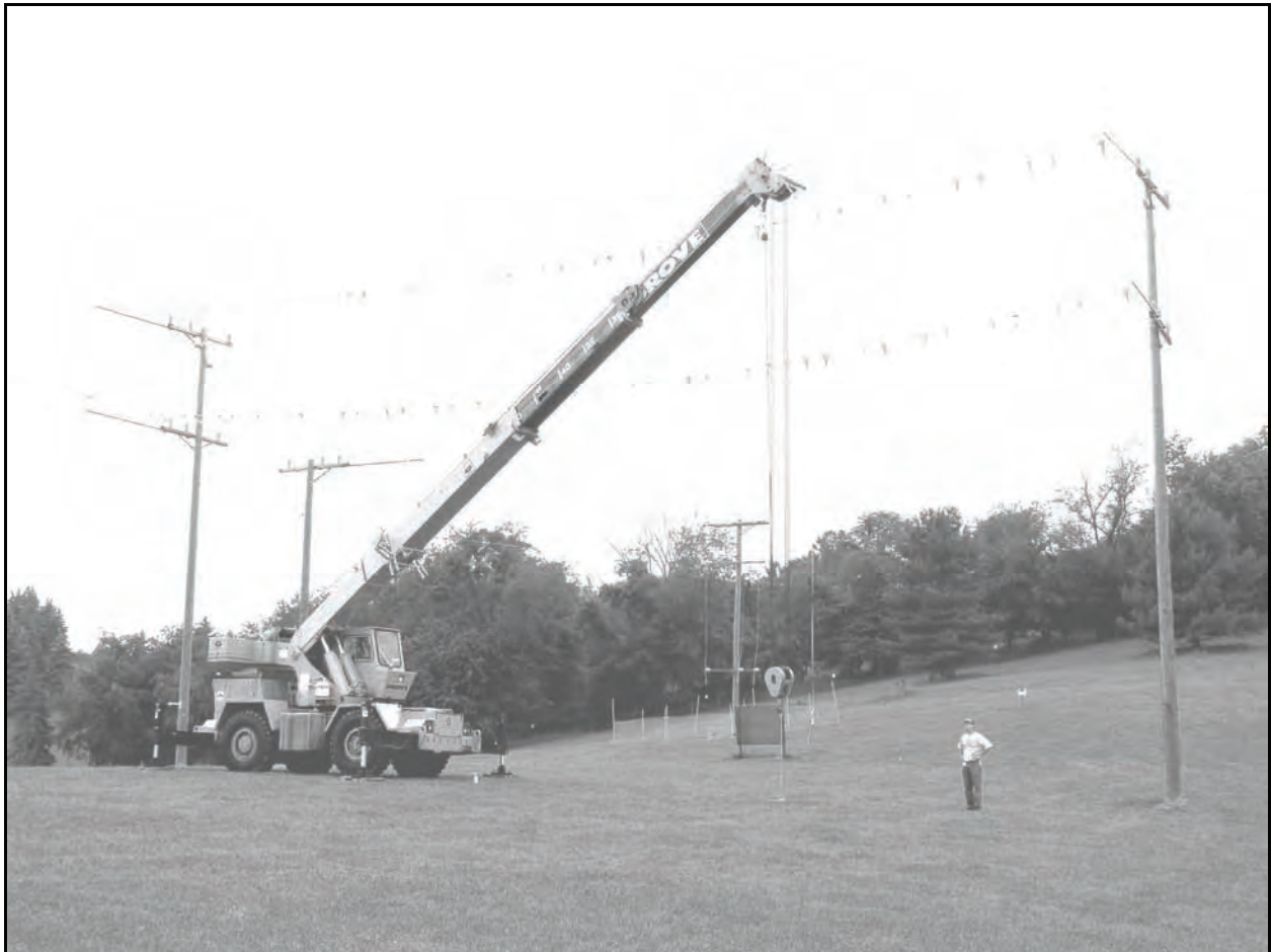
Figure 8.—Grove RT522 crane on outriggers, positioned adjacent to overhead power lines with boom at 50% extension and boom tip approximately level with lower set of lines.
