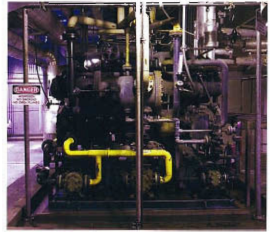
Pumps and valves below the turbine deck circulate gaseous hydrogen through the generator, cooling the rotor windings.
