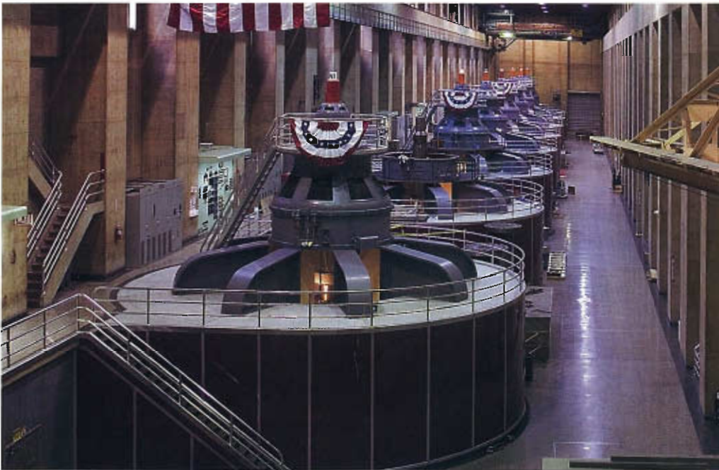
Generators at Hoover Dam are mounted with the shaft vertical. Each generator has 60 pairs of magnetic poles and turns at 60 revolutions per minute to produce 60-hertz alternating current. The eight generators seen here are on the California side of the dam; there are nine more on the Nevada side.
