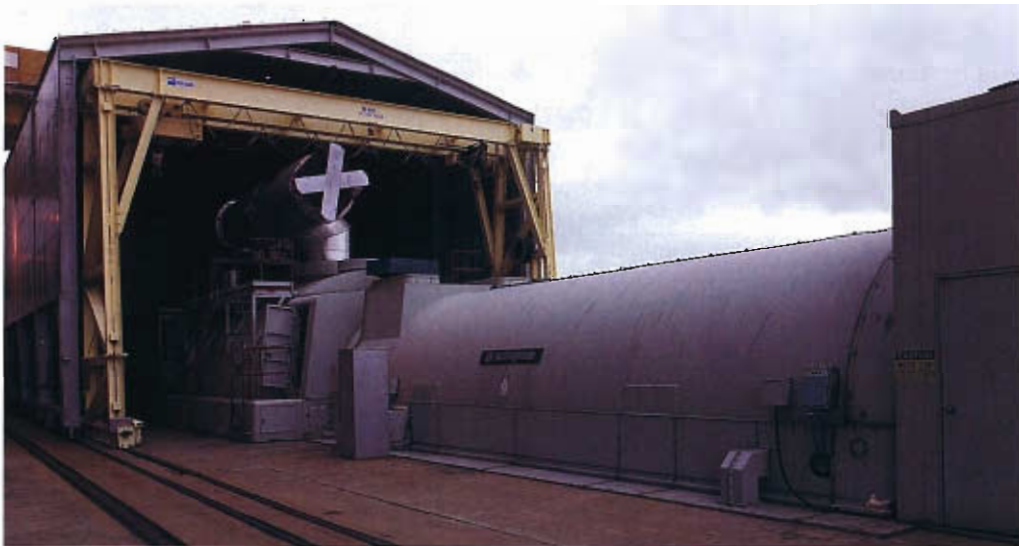
The single generator for the Mayo plant is rated at more than 750 megawatts. The generator is inside the cylindrical shroud in the foreground; the similarly shaped housing behind it is the low-pressure turbine.
