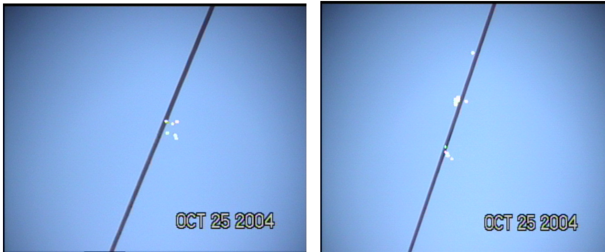
Figure 7-4 Corona observations on HTLS conductor surfaces installed in one of the field trial sites
