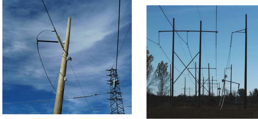
Figure 7-11 Zoom view of wooden poles carrying the Gap conductor
