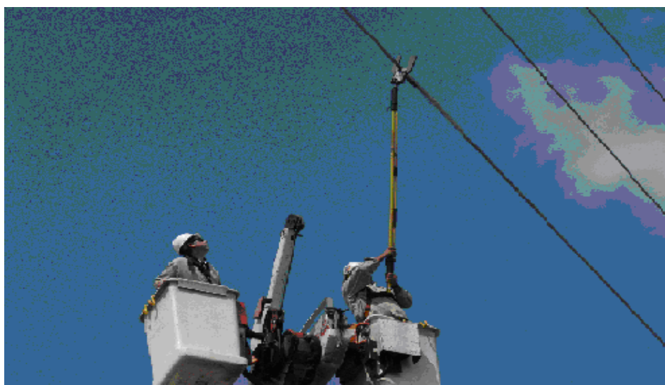
Figure 7-3 Splice resistance measurement with a Sensor Link OhmStik at the site
