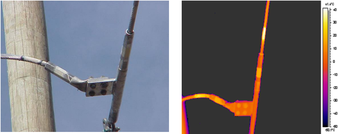
Figure 7-6 Visual and IR images of a dead-end assembly on a HTLS transmission system
