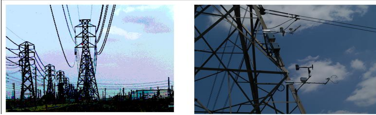
Figure 7-9 Towers and instruments installed at the CNP Energy site
